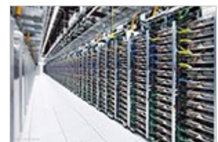
Data center Google
