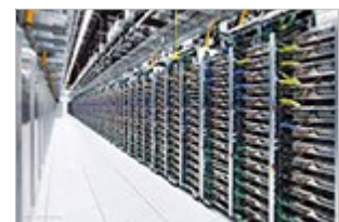
Data center Google
